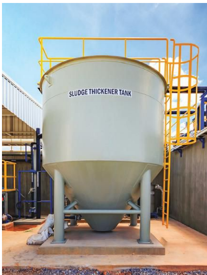
IMAGE 3: Sludge thickener tank, used to thicken the sludge for easier water extraction
